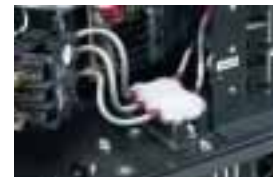
Coated Electrical Connections
